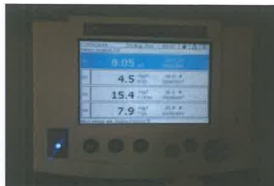
Online Monitoring at STP
